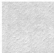
2. ORIGINAL PEBBLE AND DASH RENDER TO BE RETAINED AND RESTORED WITH SELECTED LIGHT GREY PAINT FINISH
